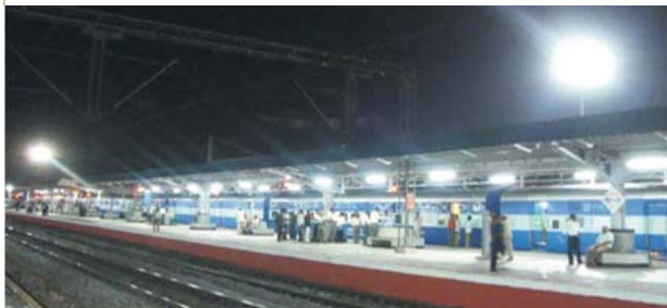
Extensive use T-5 28 watt energy efficient luminaries at stations
