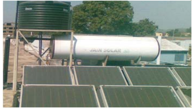
Use of Solar Water Heaters in Running Rooms, Hospitals etc.
