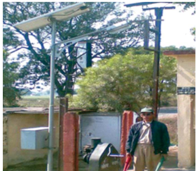
Solar Light System at Lc Gate
